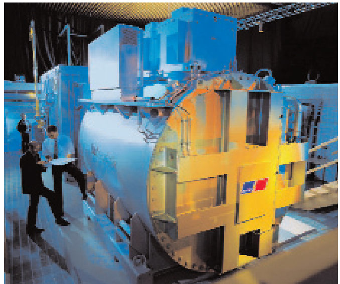
The use of fuel cells is well underway in Germany. A unit at the Rhön-Klinikum hospital in Bad Neustadt, Franconia, has reached well over 21,000 hours in operation (MTU Fuel Cells)
