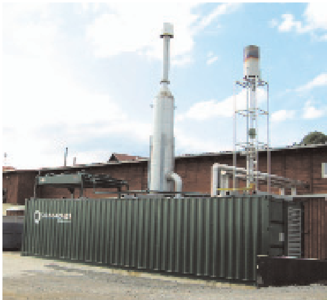
A CHP plant at Wolfring uses biogas to fuel its gas engines. The existing CHP law requires distribution system operators to buy electricity from cogeneration (GE Energy Jenbacher)
