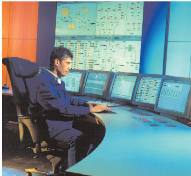
Saar Energie has taken part in one of the first approaches to develop marketable DG products in Germany (Saar Energie AG)
